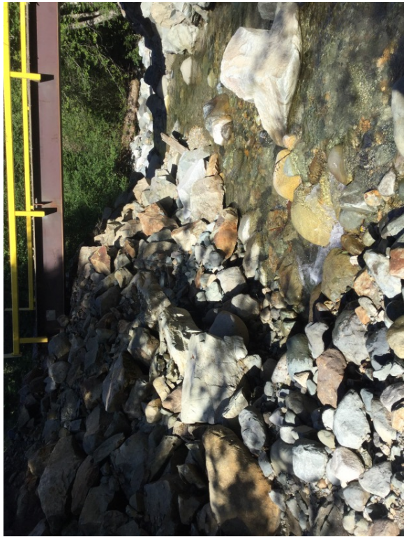
Upstream left bank riprap scour noted
